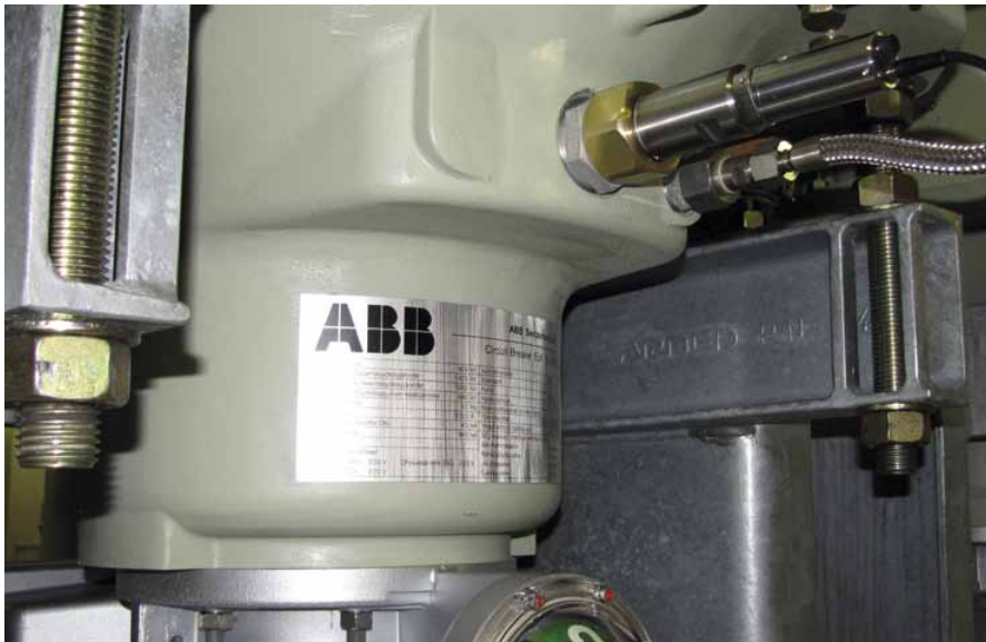
Figure 5. Installation of a dew point-pressure-temperature sensor (DPT145) directly to the main gas tank (25.3– 14.4.2010). The gas volume in the measurement cell is roughly 20 ml.
